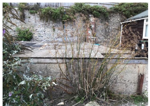
Unsafe chalet plot
