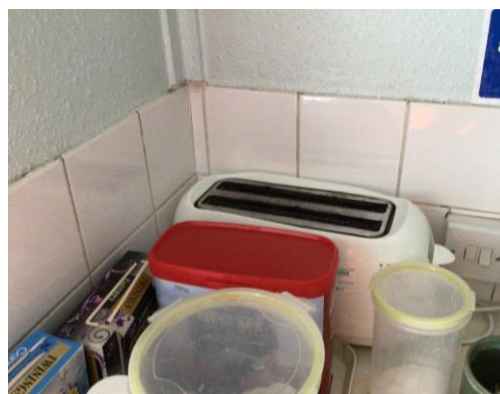
No fire blankets in kitchen areas
