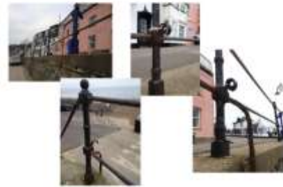
Existing Railing at Marine Parade Lyme Seafront - In need of Replacement
