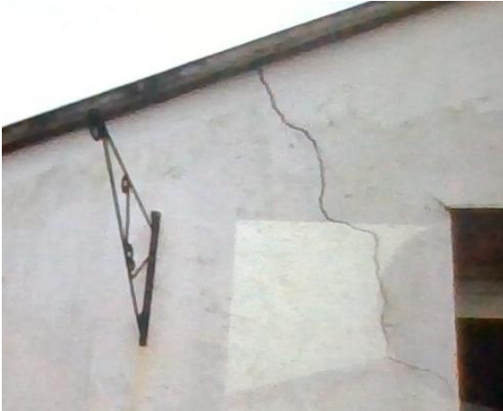
Subsidence at Cadet Hut noted
