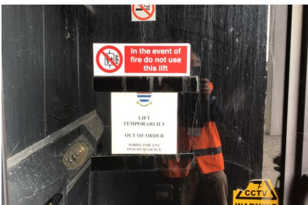
Lift out of use due to failed inspection
