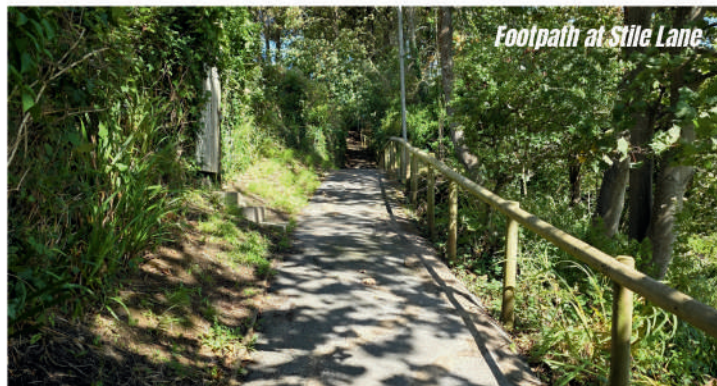
Cracks in tarmac paths
